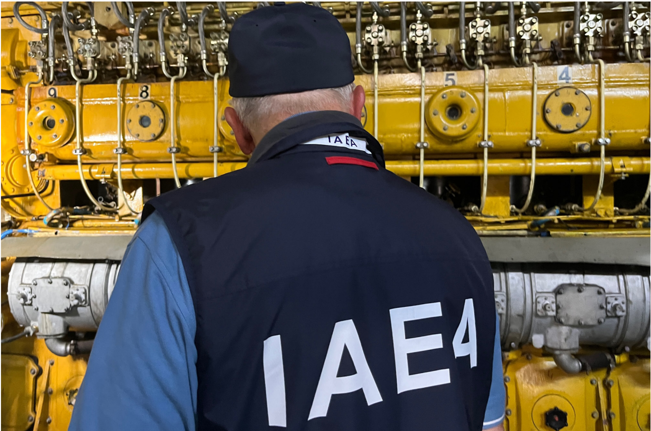
IAEA experts visiting the emergency diesel generator room of Unit 5 at the ZNPP. (Photo: IAEA)
