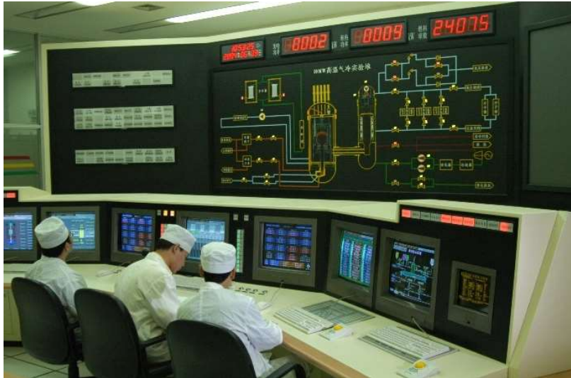
HTR-10 Control room
