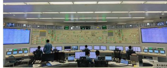
HTR-PM Main Control Room
