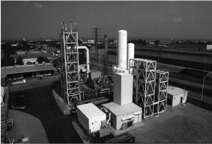
FIGURE 4.8 Prototype CIRCE plant at Hamilton, Ontario, Canada.
