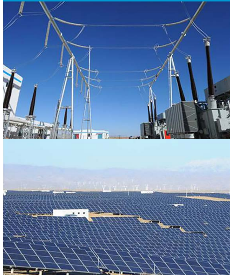
Longyangxia Hybrid Photovoltaic Power Plant Project in Qinghai province, in China: the largest single-unit grid-connected photovoltaic power station worldwide (530MW) features the complementary use of solar energy and hydro in hybrid systems (SGCC).
