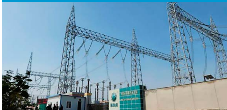
The 1,000 kV Jindongnan Nanyang-Jingmen UHV AC Pilot Project in China is 640 kilometres long and has a transforming capacity of 6,000 MVA, with a nominal voltage of 1,000 kV and the highest operation voltage of 1,100 kV (SGCC).
