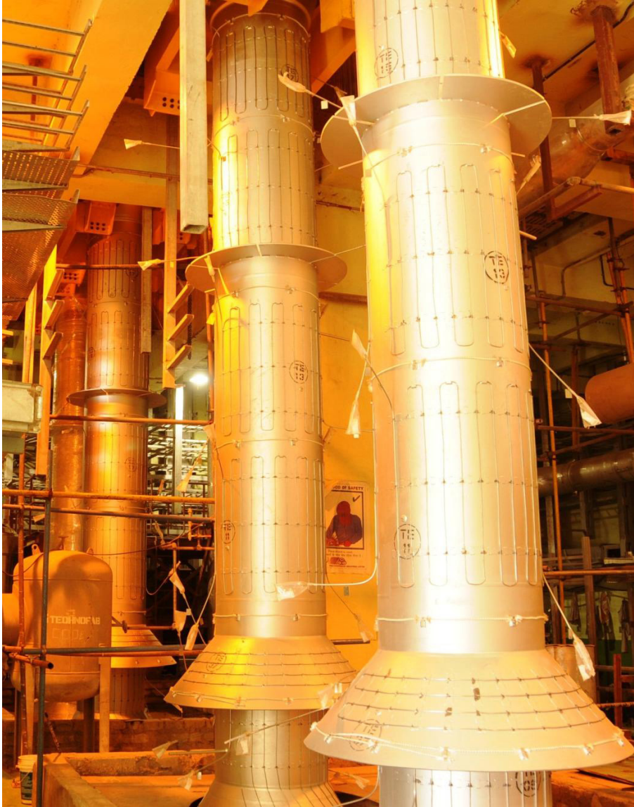
FIG. 1. Steam generators erected at the PFBR.
