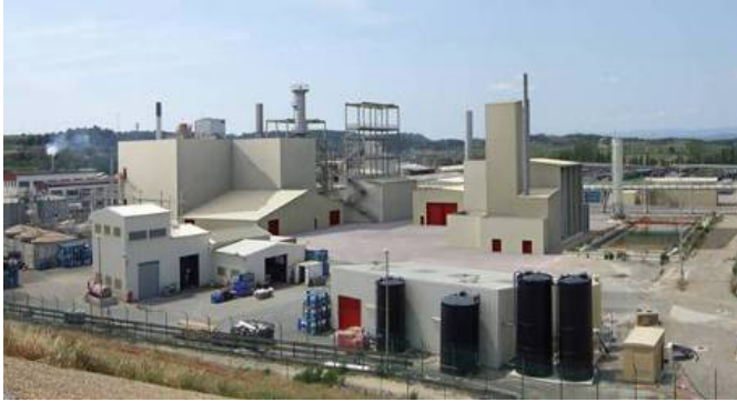
FIG. A-8. COMURHEX II conversion facility under construction in France. Gradual startup is expected in 2013–14.
