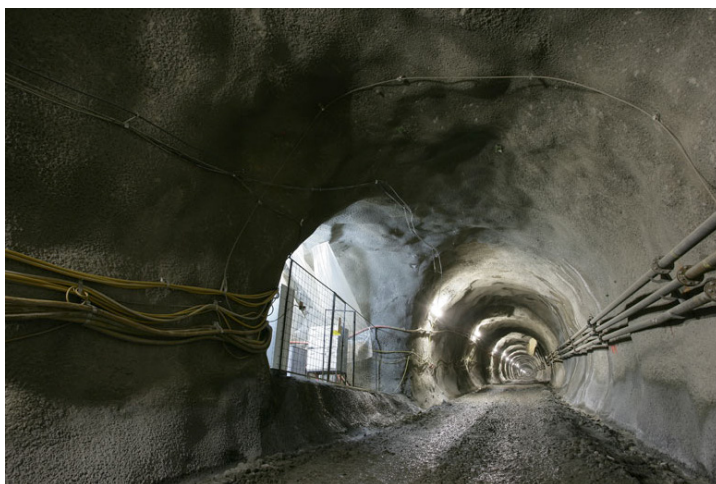
FIG. A-12. Access ramp to the national radioactive waste disposal facility at Bataapati, Hungary.
