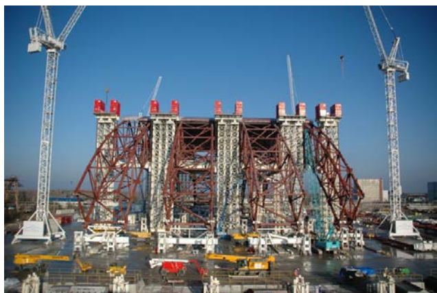
FIG. A-18. The assembly of the new safe confinement for the fourth unit at the Chernobyl NPP (Photograph courtesy of Chernobyl NPP).
