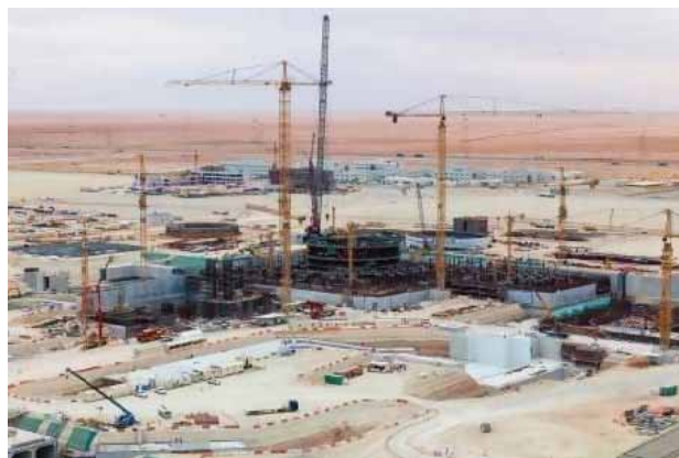
Construction continues at the site of the UAE's first nuclear-power plant at Barakah-1 in the Western Region. Photo courtesy Emirates Nuclear Energy Corporation
