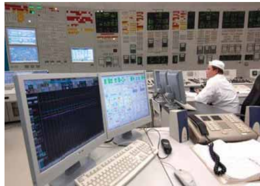
Control Room of Reactor Leningrad (RBMK or LGWR)
